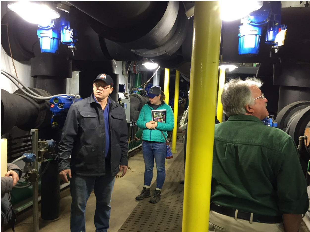
City of Dunkirk Water Treatment Plant Operator Bob Lowrie describes recent upgrades to the Water Treatment Facility to LEMC members.
